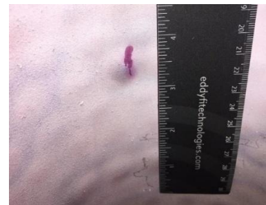
Figure 3: Condition of the pipe internal surface
