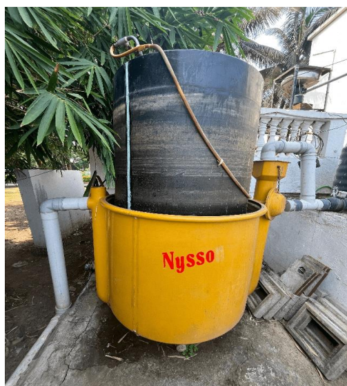
Figure 2. Secondary digester containing the floating-head drum at maximum capacity of gas production. PVC gas outlet pipe and HDPE primary containment clearly seen. Corrosion problem not observed because of polymer composite design.
