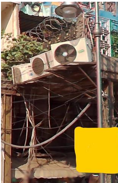
Figure 1. Cluttered electrical wiring.
