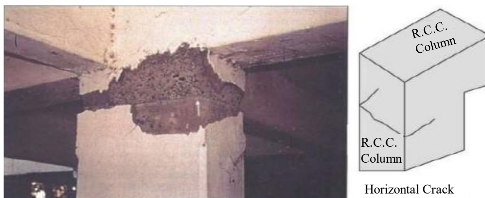
Figure 8. Horizontal Cracks Due to Moment Resistance.
