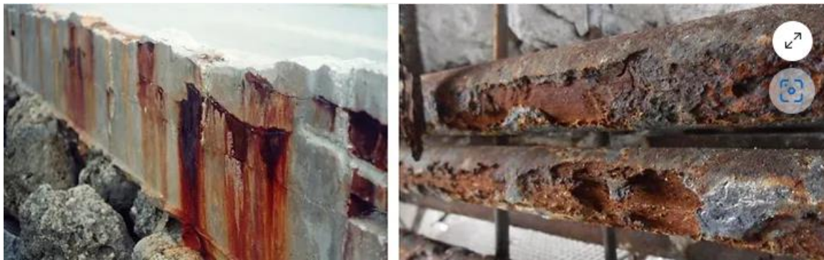
Figure 6. Chloride Attack Effects over Concrete and Reinforcement Steel.
