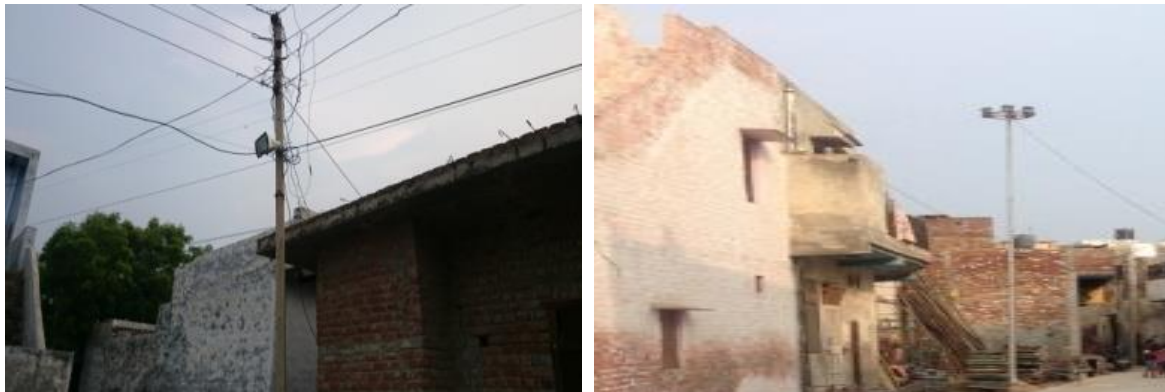
Figure 20. Condition of streetlight in Barauli Village.
