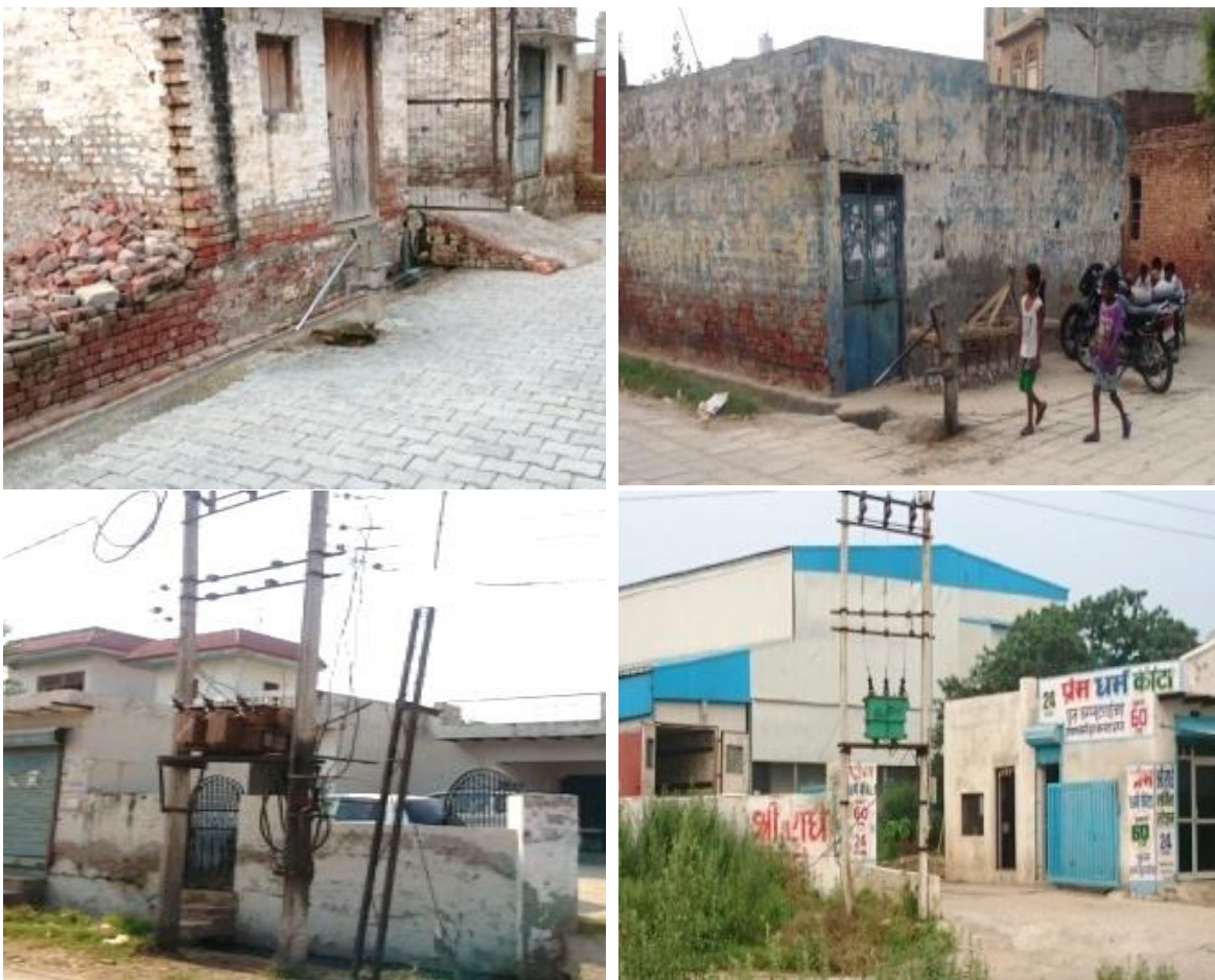
Figure 19. Condition of transformer in Barauli Village.
