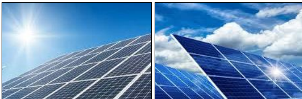
Figure 2. Roof top solar panel.
