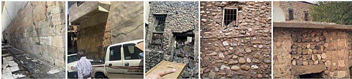
Figure 11. Wall cover typology reshaped. Natural stone, stream stone and concrete block.
