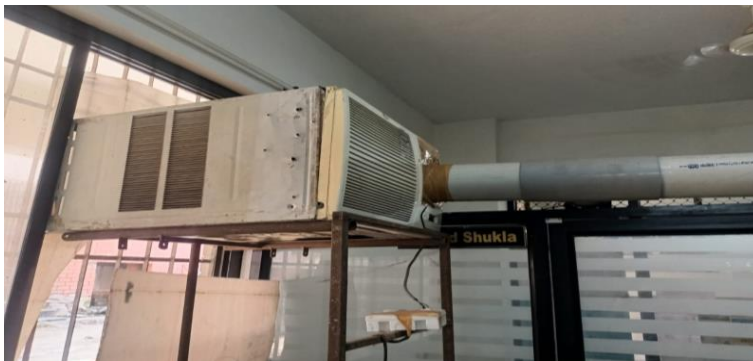
Figure 1. Installed 1.5 T window AC.
