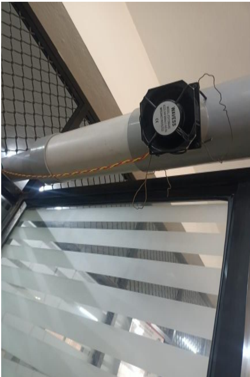
Figure 3. Air circulation controlling system using a suction fan.
