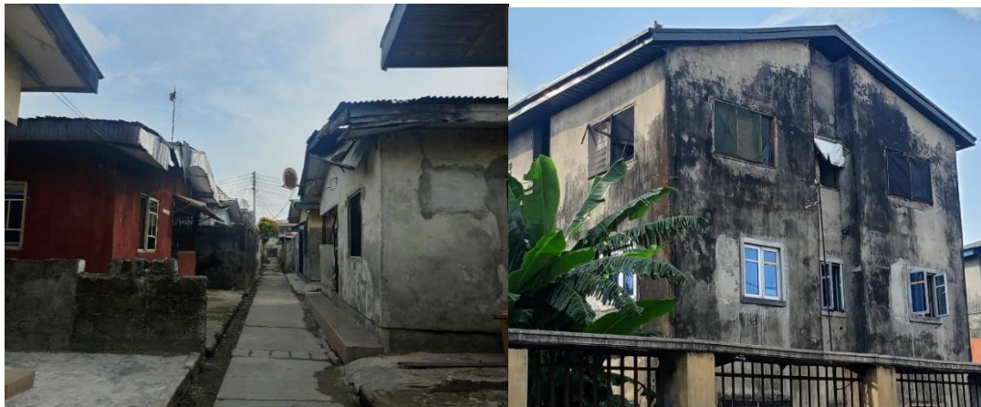
Figure 5. Showing roof decay and impact on other component in port harcourt township and inadequate eave cover with a corresponding decay on external walls in mgbunbungwu neighbourhood.
