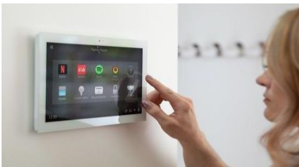
Figure 12. Touch screen security system. Source: https://pin.it/SU1YwnOnP
