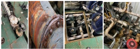
Figure 2: Engine room Pipe Line (Corrosion Identified Area)
