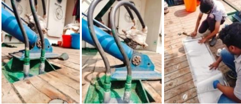
Figure 1: Side A-Frame Pipe Line (Corrosion Identified Area)
