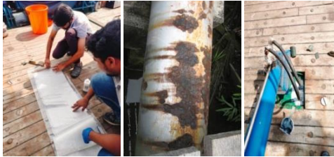
Figure 5. Coating on corroded pipeline
