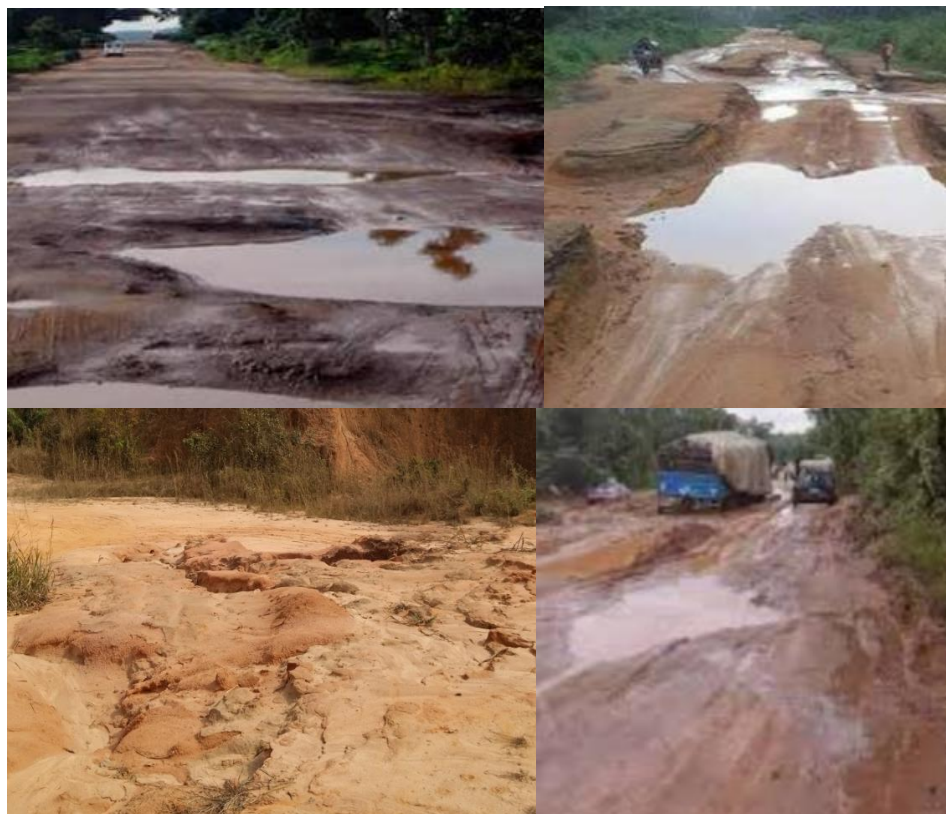
Figure 2. Some failed sections of the A123 Ilorin – Lokoja federal highway.
