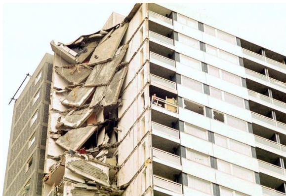
Figure 1. Progressive collapse of building.
