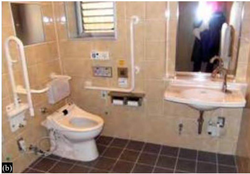
Figure 15. (a) and (b) Inclusive restrooms.
