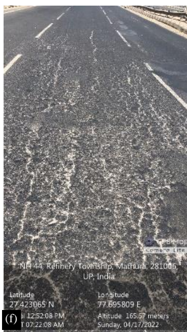
Figure 2. (f) Represents alligator cracking with low severity pot holes.
