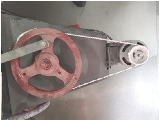
Figure 7. Pulley drive for conveyor.
