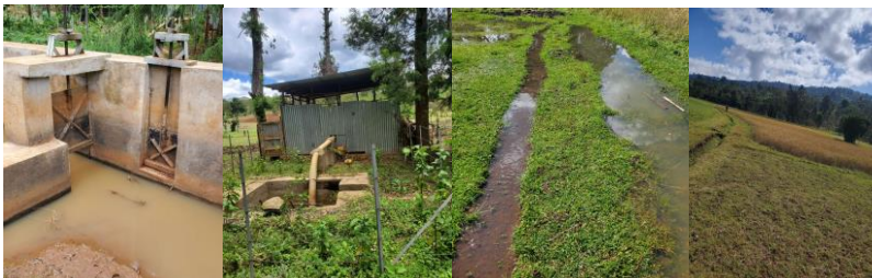
Figure 5. Head work and motor pump irrigation scheme in Batigotu kebele.
