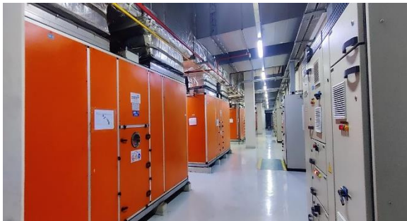
Figure 1. Depicts a typical basic air handling unit located in the mechanical room within the facility.
