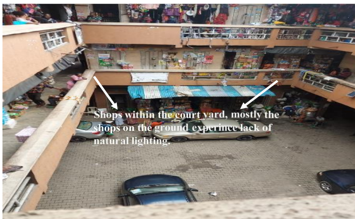
Figure 4. Image showing shops within the court yard of the market building that lacks natural lighting of Rumu-Woji market.
