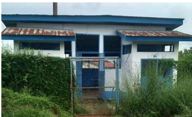
Figure 7. Waste storage facility at the Kambia Government Hospital.
