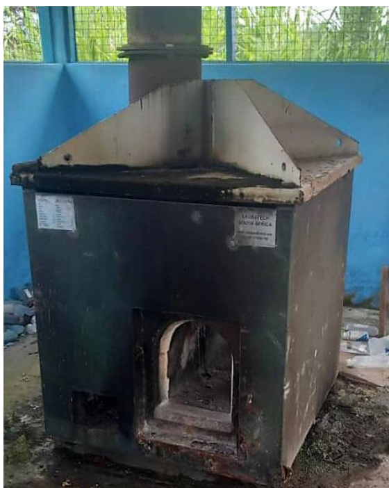
Figure 8. Kambia Government Hospital's non-functional incinerator.
