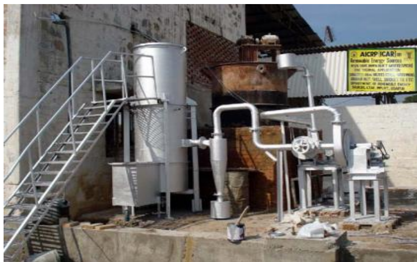
Figure 4. Gasifier installed at M/s Phosphate India Pvt. Ltd., Udaipur.
