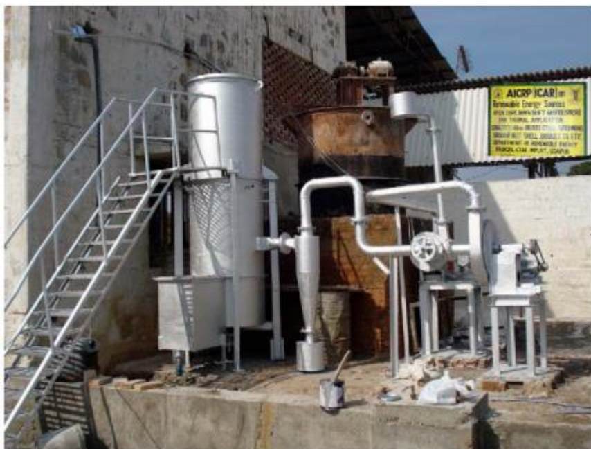
Figure 4. Gasifier installed at M/s Phosphate India Pvt. Ltd., Udaipur.
