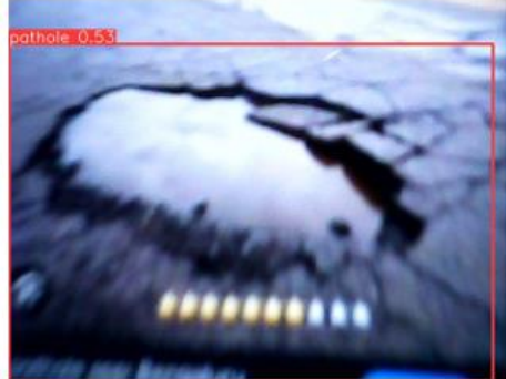
Figure 6: Pothole detected by YOLOv5
