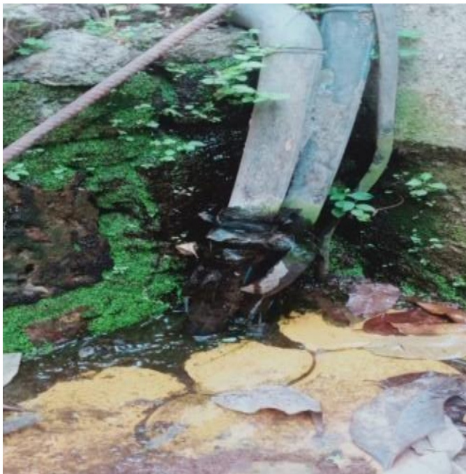
Figure 10. The location is below the main water tank.
