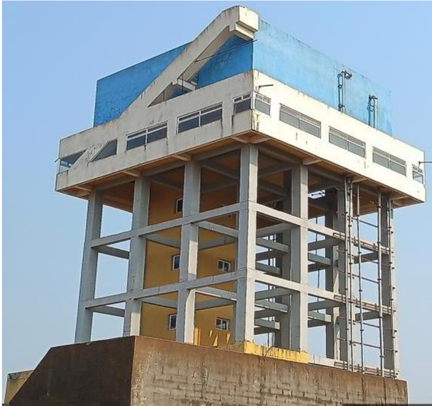
Figure 3. The capacity of the storage tank is 9 lakh liters.
