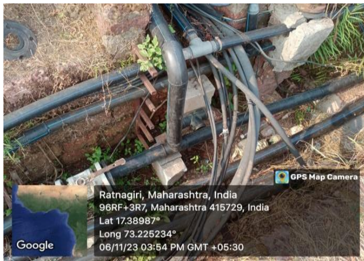
Figure 7. Joint machine domestic water consumption.
