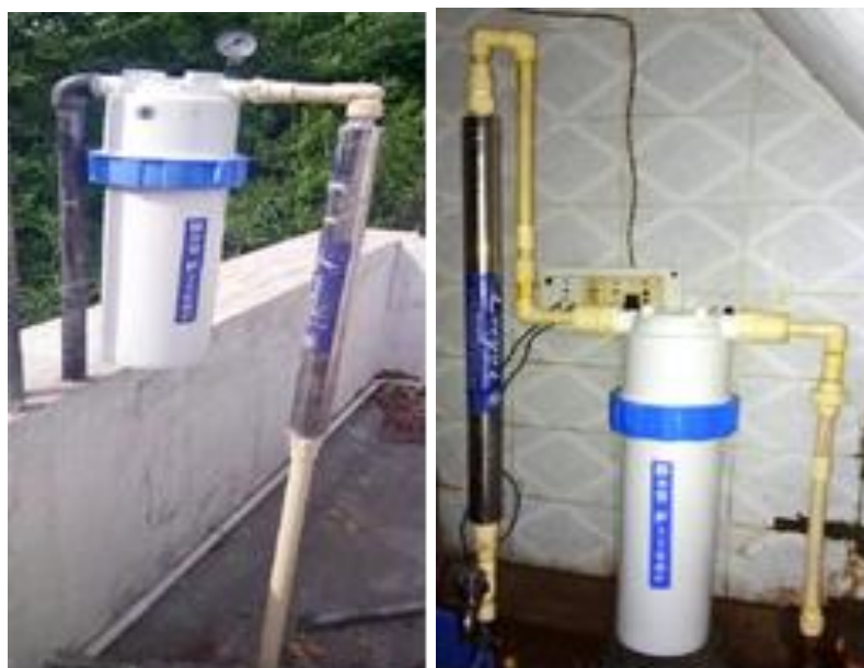
Figure 1. Outdoor and Indoor Setup for water treatment by Implosion Technique.
