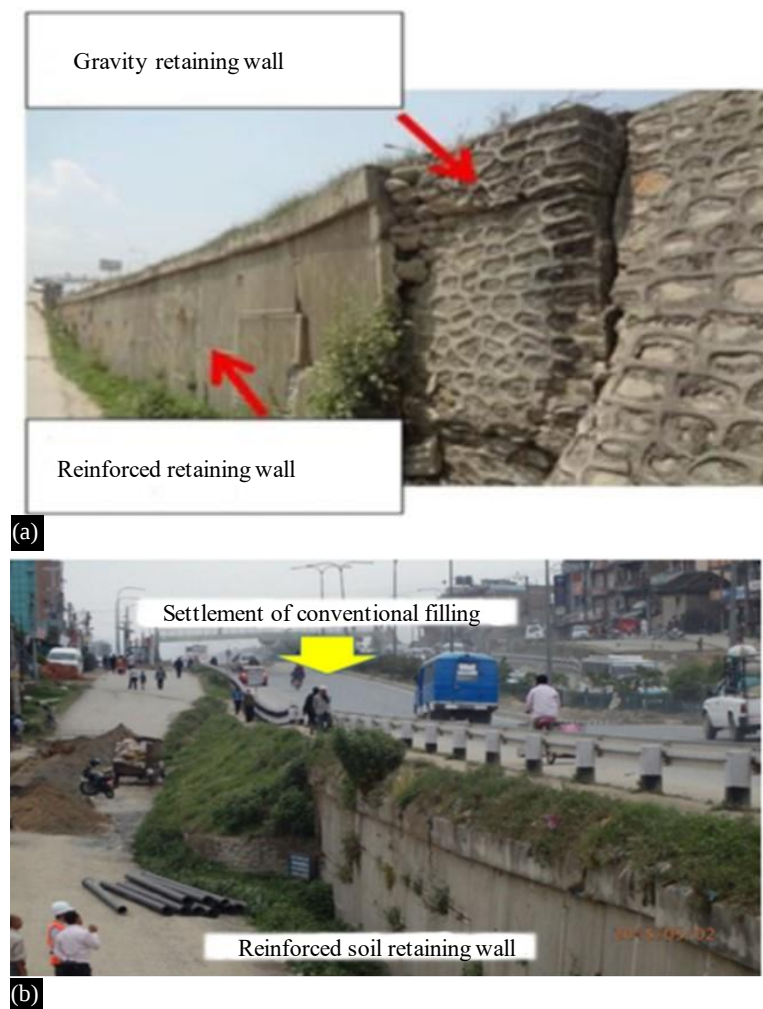
Figure 1. Various scenario of reinforced soil wall failure (a) Nepal earthquake in 2015 (Okamura et al., 2015) (b) Gorkha Nepal earthquake in 2015 (Chiaro et al., 2015)
