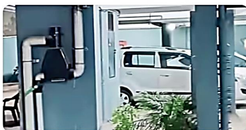
Rainwater harvesting system at Windsor Avenue building in Wanowrie. The system helped society become tanker-free
