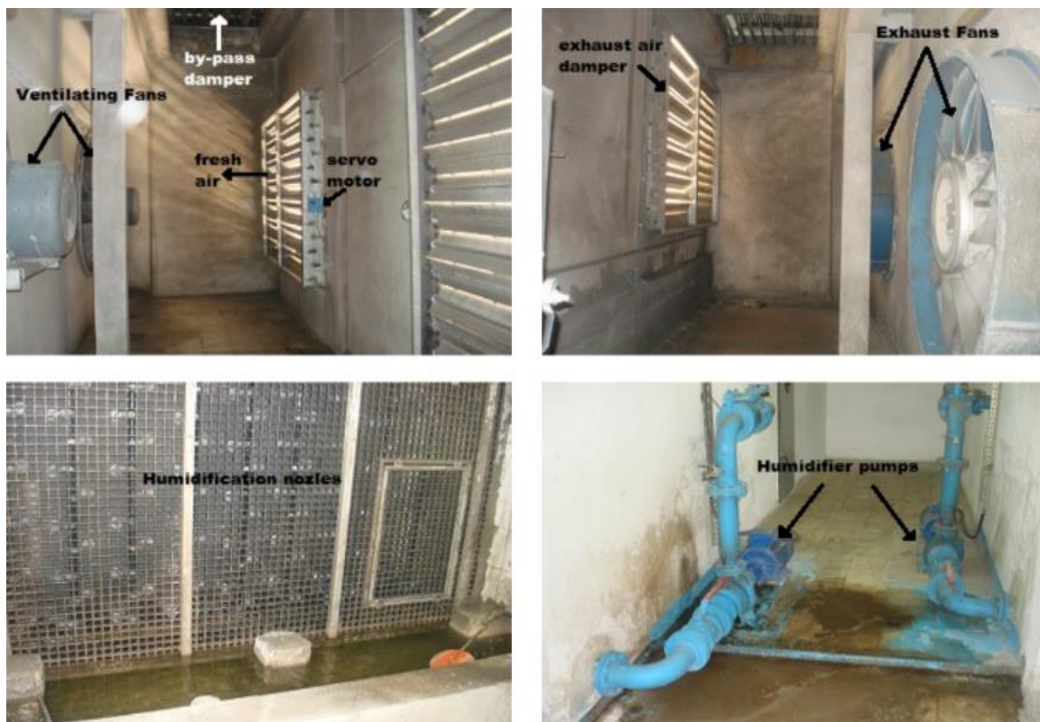
Figure 4. General view of HVAC unit of controlled system.
