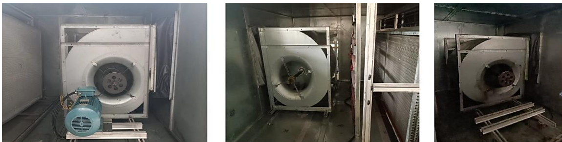
Figure 4. Blower type Fan Before Retrofitting of EC + Fan.
