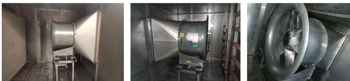
Figure 5. After Retrofitting of EC + Fan.
