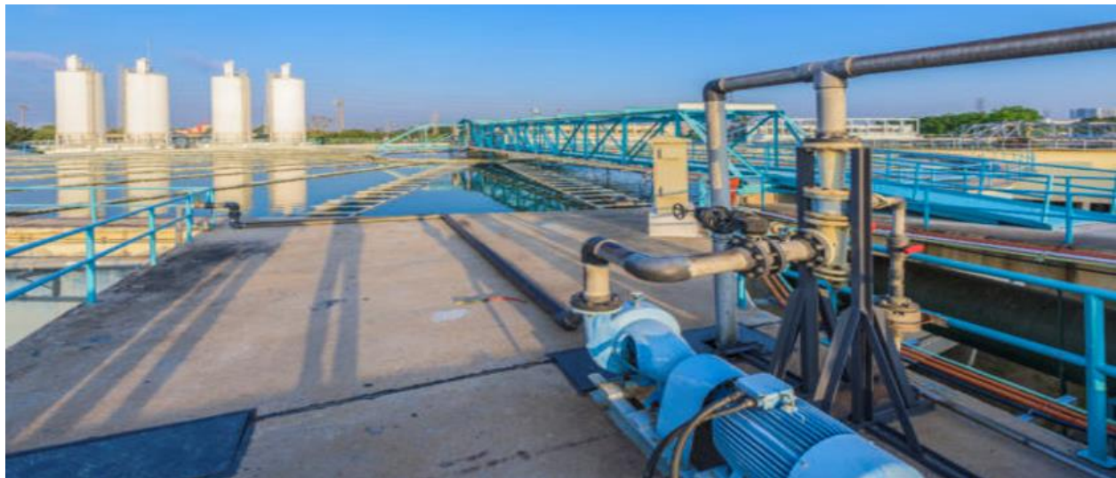
Figure 2: Typical Water Treatment Plant
