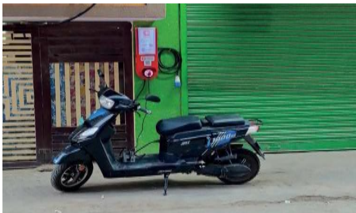
Figure 2. Presentation of the charging station.
